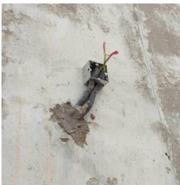
Figure 2.3 This implementation of the box is correct, but the pipes are wrong. It is assumed that the pipes are broken inside the wall like an interior work.
