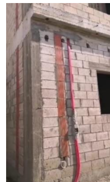
Figure 2.4 It is an error to tape the box with cement instead of nails, and to not break to the pipes inside the wall. Correct: Nail the box to the wall and insert the pipes.
